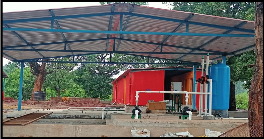
Photo # 9(A) Sewage Treatment Plant (80 KL) at base camp
